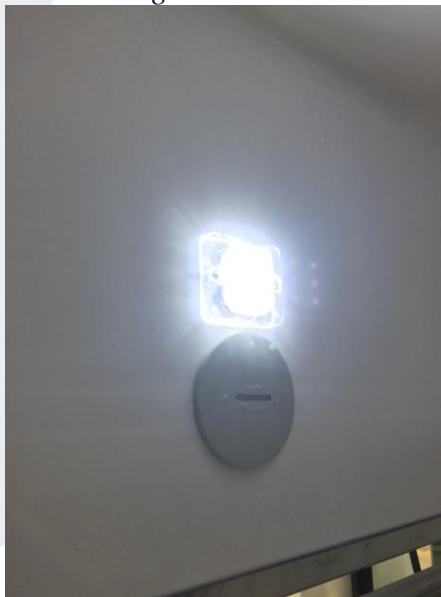
internal led lights above the side doors
