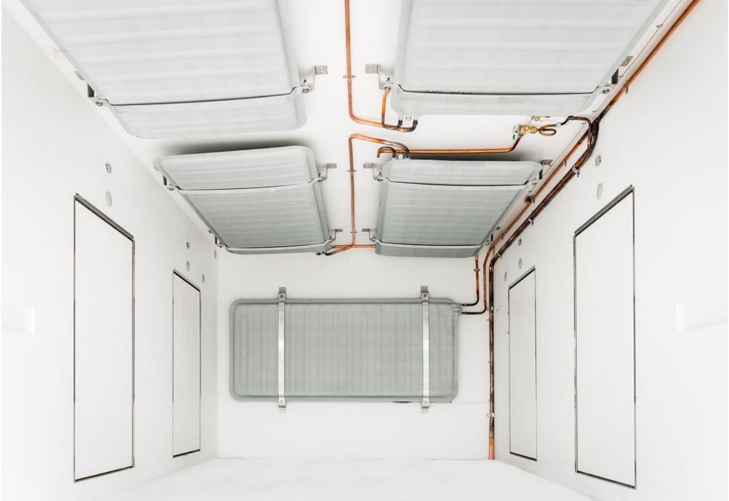
internal eutectic plates and copper piping view
